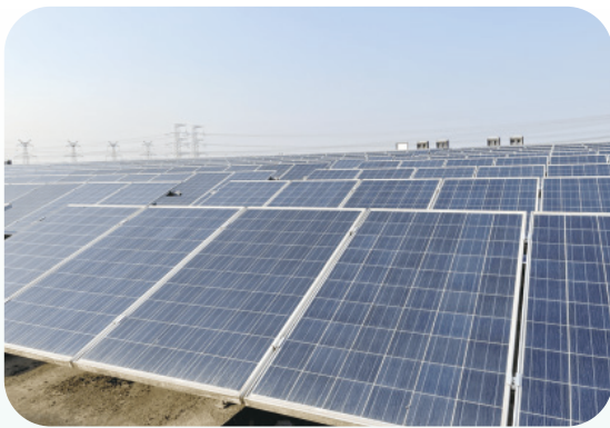
^ Joyoung photovoltaic power generation facilities
